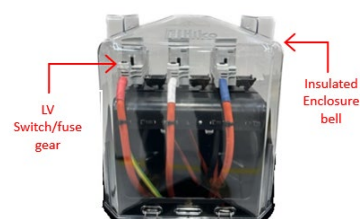
Bell and Internal fuse gear on insulated stand
