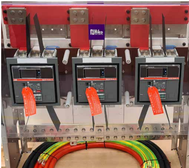
Incomer Circuit Breaker with 2 Feeder Circuits Breaker Frame
