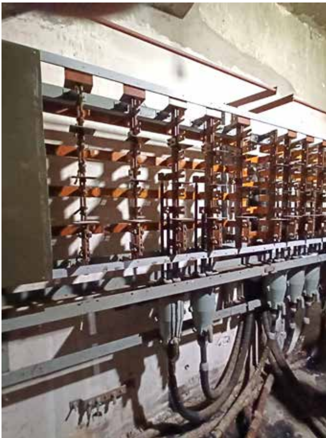
Outdated existing fuse rack system upgrade
