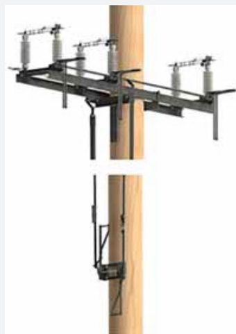
Mid Pole, Side Break Switch with manual operating handle and associated Earth Switch.
