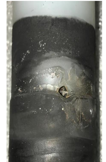
PD in service. Break Down in cable insulation
