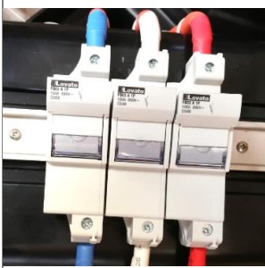
Plugs can be removed to gain access for testing
